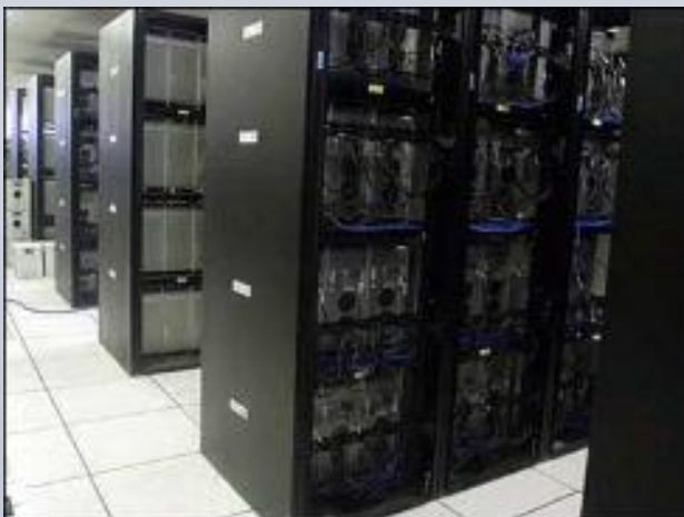
System X at the Virginia Tech CRC
